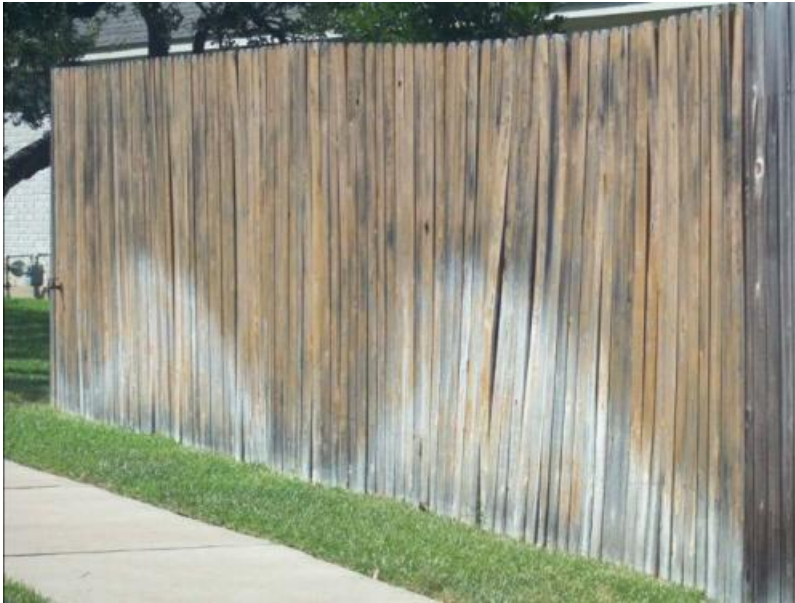
Example 3: Violations include washed-out stain, warped pickets, and a leaning section of fence.
