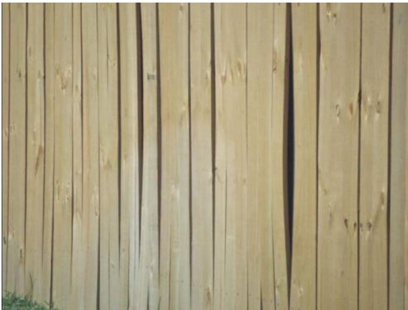
Example 2: Boards warped beyond acceptable standards.
