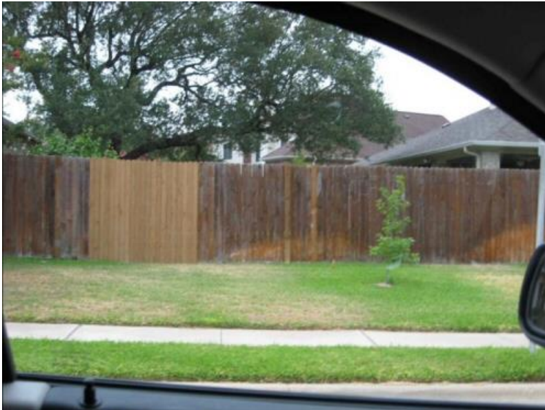
Example 4: Washed-out stain and new pickets without stain.
